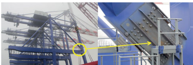
Fig. 5. Examples of anti-seismic devices' installation on single bracing support container crane
