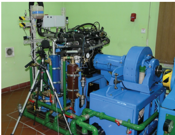
Fig. 4. View of the engine installed on the research rig
