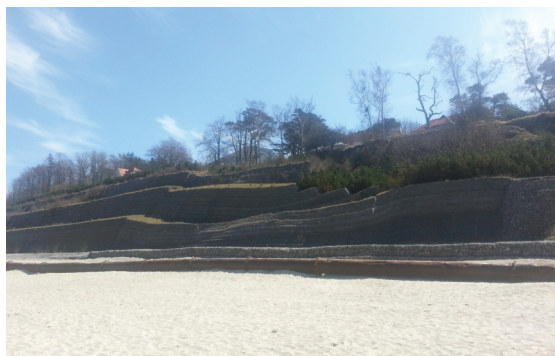
Fig. 3. Deformations of the cliff protection structure made of reinforced ground and gabions (2014) [8]
