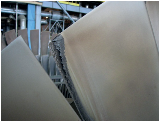
Fig. 4. Leading edge damage patterns observed in the 225 MW turbine last stage rotor blade system
