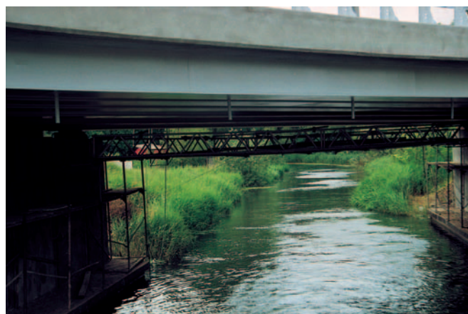
Photo 5. (J. Kulczyk, R. Werszko) A repair of the road bridge over the Upper Noteć Canal. The changes being introduced during the repair work are expected rather to remove the existing obstacles for ship traffic than to cause more troubles .
