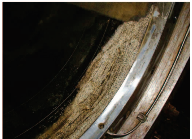
Fig. 3. Damage of a composite bush, resulting from edge thrust resulting from skew position of shaft axis (up); during repair the damaged edge was grinded to avoid cracks and delamination of the composite (down)
