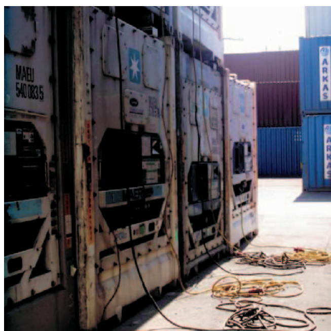
Fig. 2. Reefer containers cut-off from the electricity supply source on store place
