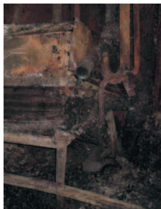
Fig. 12. Open ducts of air cooling system (the view after fire accident)
