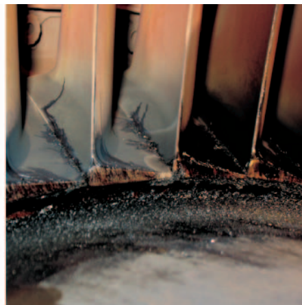
6th stage of propulsion turbine of LM-2500 engine – traces of carbon deposit on rotor blade surface
