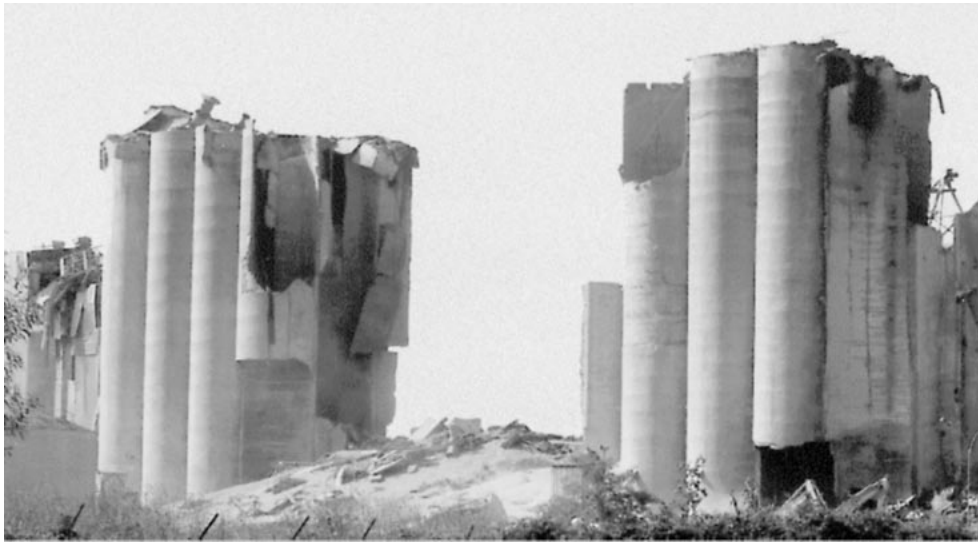
Figure 1. Silo plant in Blaye, France, after a dust explosion (photo: J. Steiner [1])
