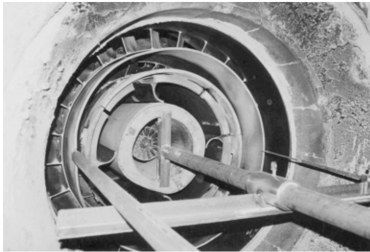
Figure 2. A Babcock Energy burner during measurements of the velocity components in the OP-230 boiler No. 10, Heat and Power Plant in Gdansk
